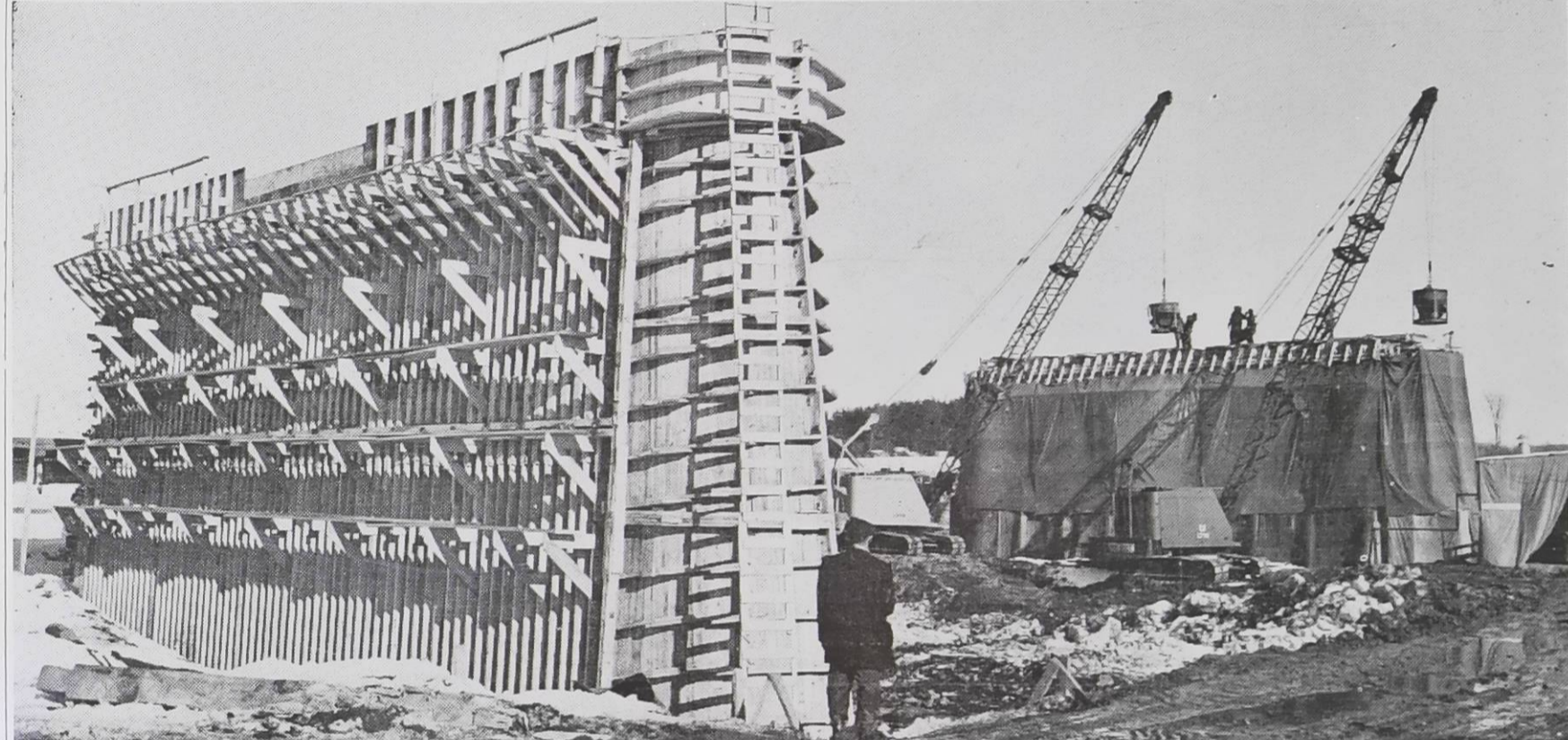
The most active spot in Drummondville for the time being seems to be St. Francis river where a new bridge is under construction. Around 100 men are working there. Above, a general view of the building area. Below appears the second pillar out of seven which will support the new steel bridge to be laid over the river.
