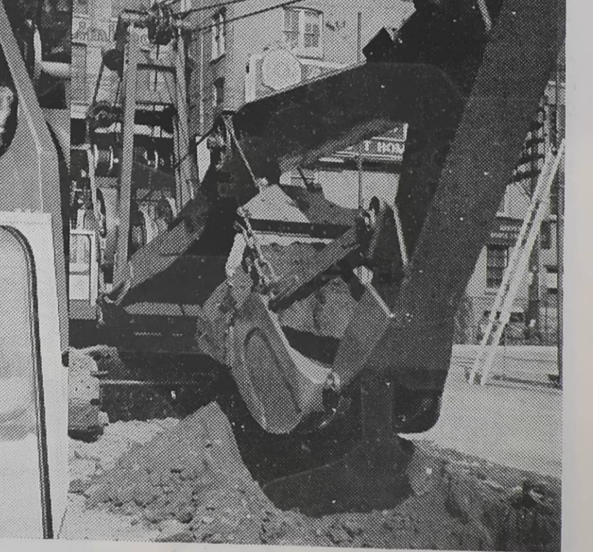
N. R. Crump, president of the Canadian Pacific Railway, pulls the switch of the steam shovel that turned the sod recently for the new $10,000,000 400-room addition to the Royal York Hotel in Toronto. Scheduled for completion in 1958, the 17-storey addition will make the Royal York Hotel the largest in the Commonwealth with 1,600 rooms. In attendance at the ceremony were Hon. Leslie Frost, Premier of Ontario, Fred G. Gardner, Chairman of the Board of Metropolitan Toronto, Mayor Nathan Phillips of Toronto and Hon. Bryan A. Cathcart, M.L.A., Minister of Travel and Publicity, Province of Ont.
